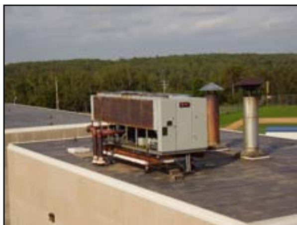
HVAC - Dehumidification Chiller and Piping Mains
