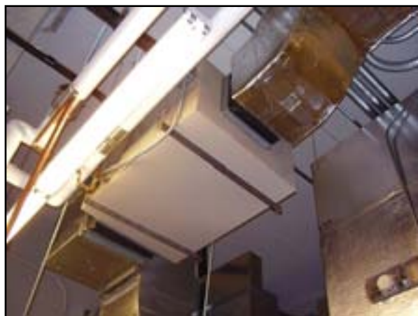
HVAC: Upgrade Ventilation in Classroom Areas
