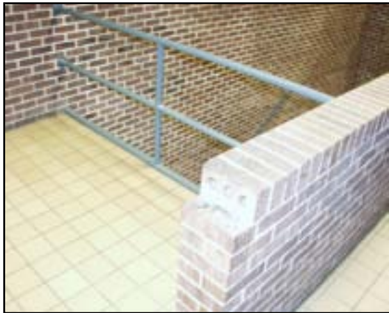
Stairs: Replace Guardrails at Top of All Stairs
