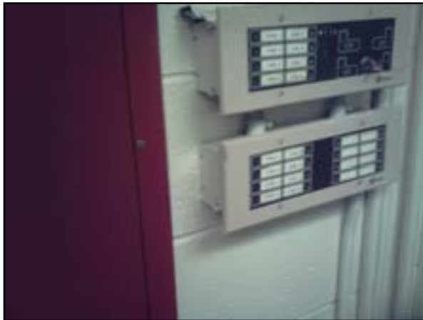
Fire Alarm Systems: Outdated System
