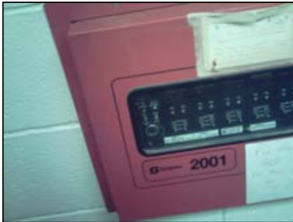
Fire Alarm Systems: Outdated System
