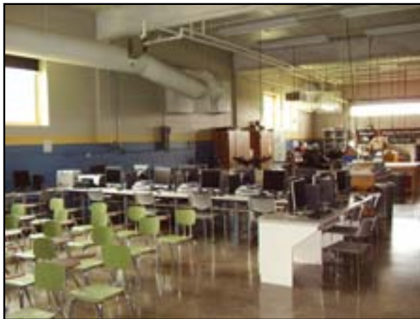
HVAC: Upgrade Ventilation in Graphic Arts and Small Engine Areas
