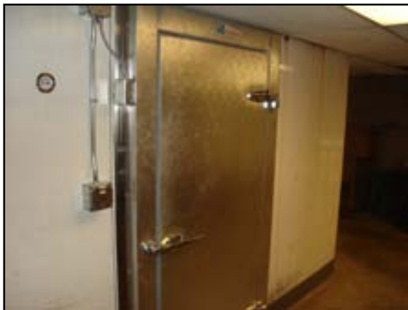
Other Equipment - Walk-In Freezer Basement
