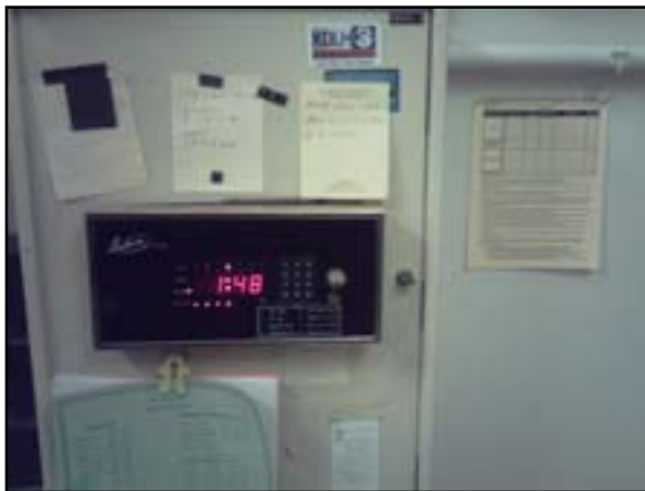
Communication and Security: Clock System
