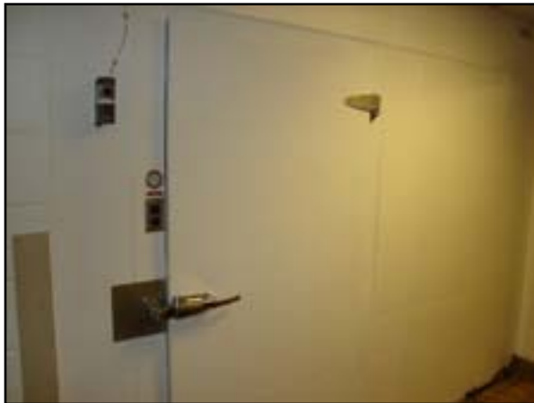
Other Equipment - Walk-In Freezer Prep Area
