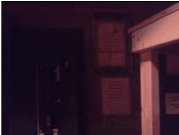
Electrical Distribution: Insufficient Capacity
