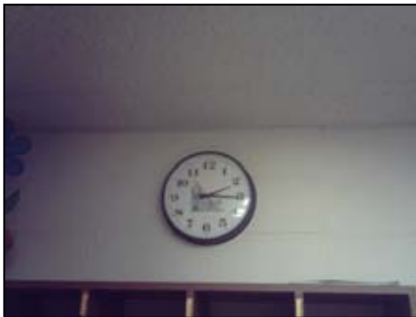
Communication and Security: Clock System
