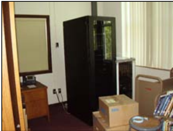
HVAC: Add Cooling Capability to IT Data Room
