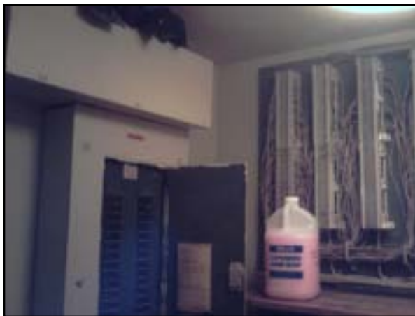
Electrical Distribution: Insufficient Capacity
