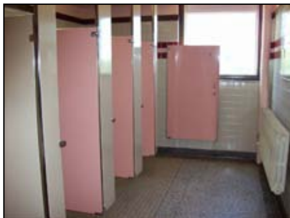
Fittings: Toilet Partitions
