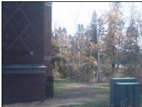
Emergency Power Distribution: Generator Backup
