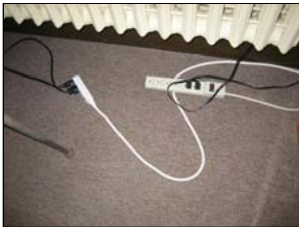
Wiring Devices: Insufficient Receptacles
