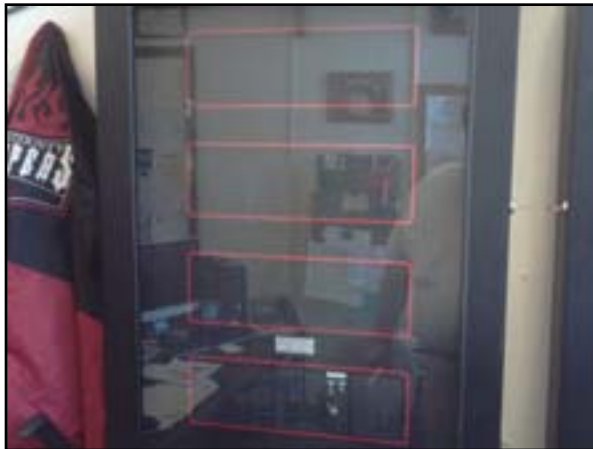
Fire Alarm Systems: Outdated System
