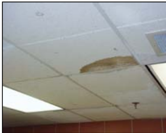
Ceiling Finishes: Replace Damaged Ceiling Tile
