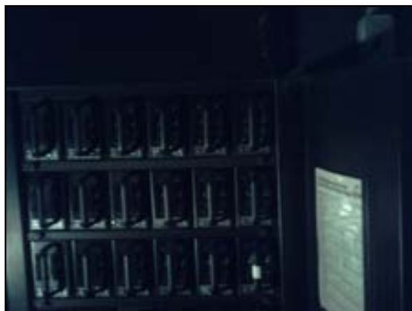
Lighting Equipment: Dimming System
