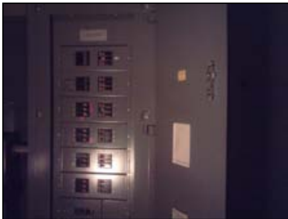
Electrical Distribution: Insufficient Capacity
