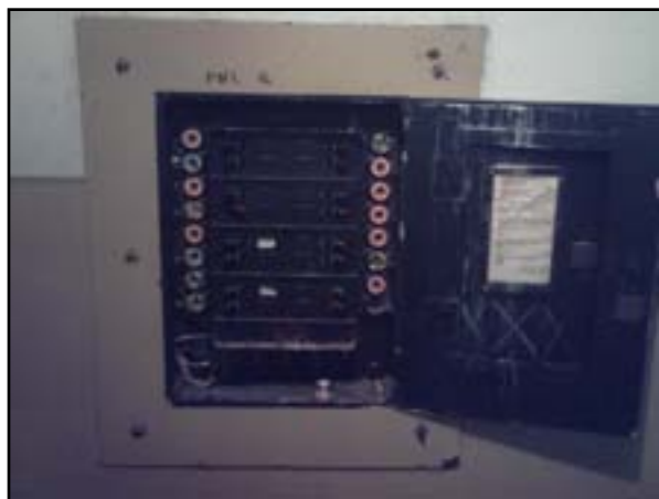
Electrical Distribution: Outdated Panels
