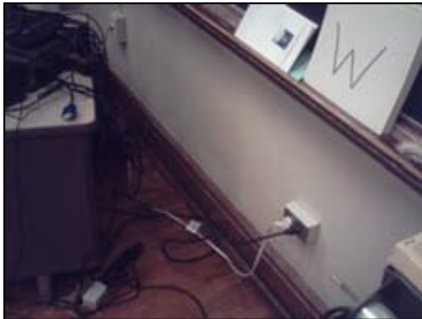
Wiring Devices: Insufficient Receptacles
