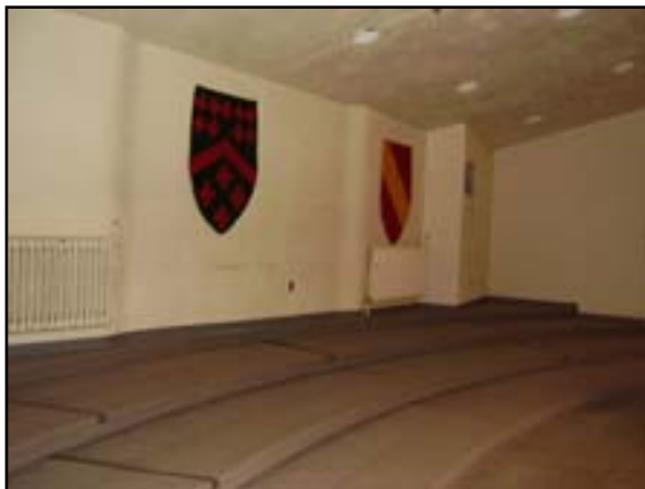
HVAC: Upgrade Ventilation and Add Dehumidification 1958 Music Additon
