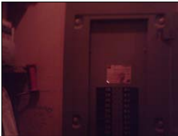
Electrical Distribution: Insufficient Capacity
