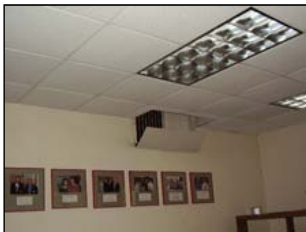
HVAC: Replace Ventilation All Floors 1926 Building Classrooms and Auditorium
