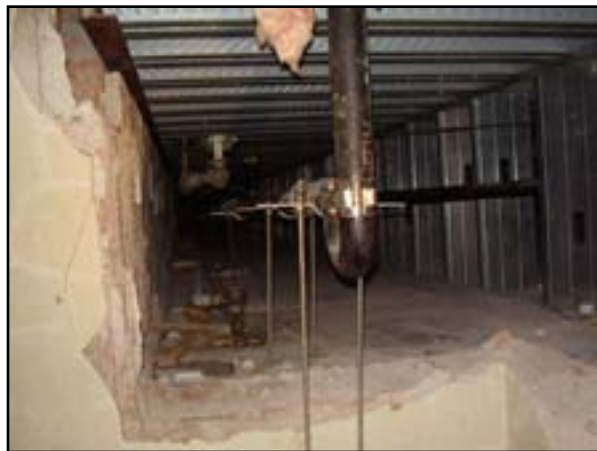
HVAC: Provide Negative Pressure in Crawlspace/Tunnels
