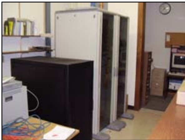
HVAC: Add Cooling Capability to IT Data Rooms
