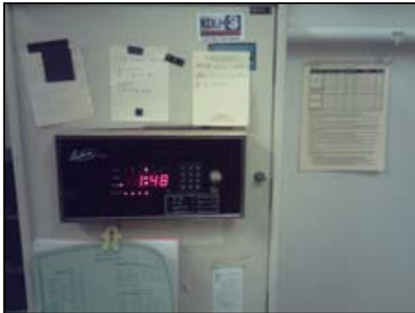
Communications and Security: Clock System
