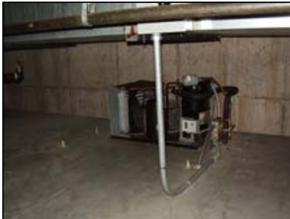
HVAC: Remote Condenser Heat Removal
