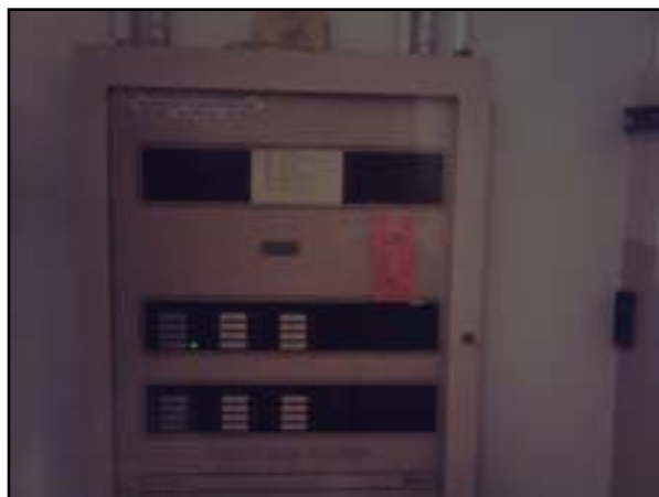
Fire Alarm Systems: Outdated System
