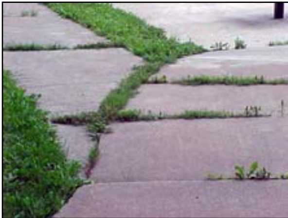
Site Improvements: Accessibility
