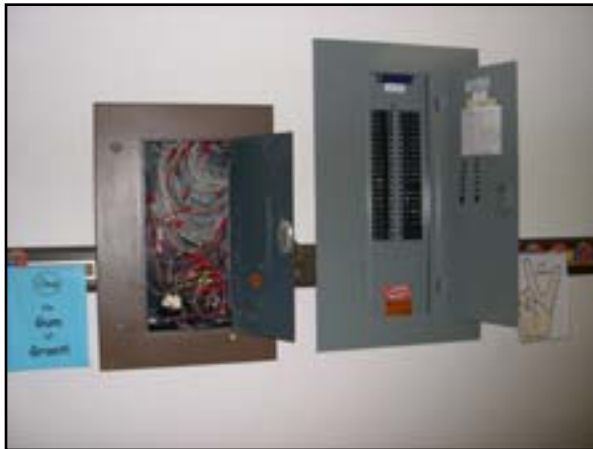
Electrical Distribution: Insufficient Capacity
