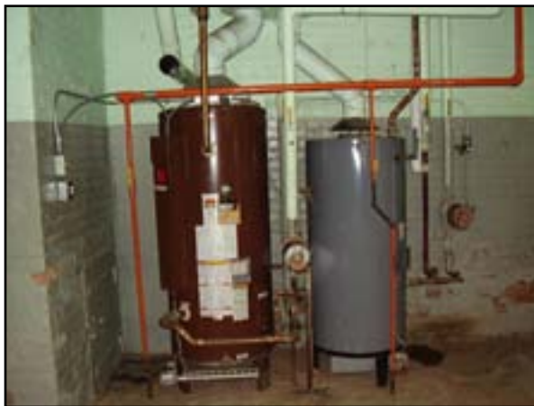
Plumbing: Add Dometic Water Heat Exchanger
