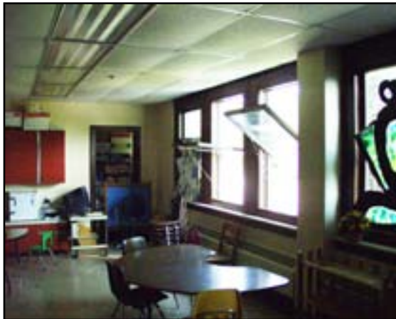
Ceiling Finishes: Replace All Suspended Acoustical Board Ceilings
