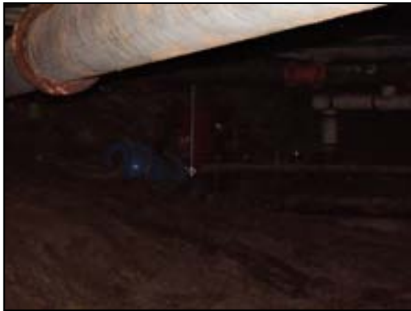
HVAC: Provide Negative Pressure in Crawlspace/Tunnels
