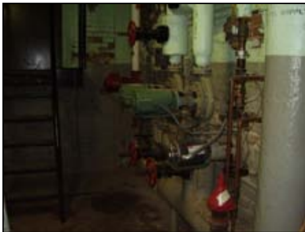
HVAC: Add Propylene Glycol to Heating System
