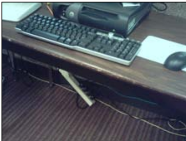
Wiring Devices: Insufficient Receptacles
