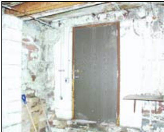
Exterior Doors: Replace Basement Door at Main Entrance
