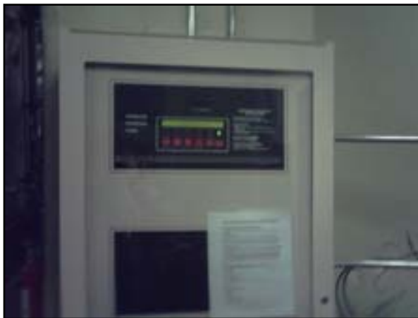
Fire Alarm Systems: Outdated System
