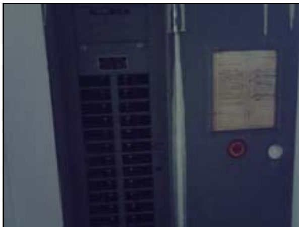
Electrical Distribution: Insufficient Capacity
