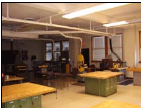
HVAC - Upgrade Ventilation and Replace Wood Shop Dust Collector and Upgrade Weld Hood Exhaust
