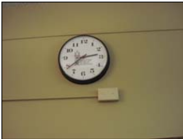
Communication and Security: Clock System
