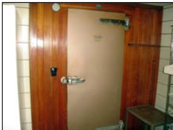
Other Equipment - Walk-In Cooler
