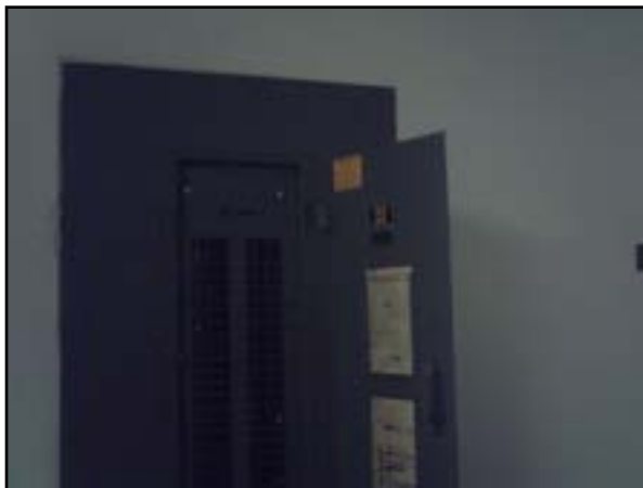
Electrical Distribution: Insufficient Capacity
