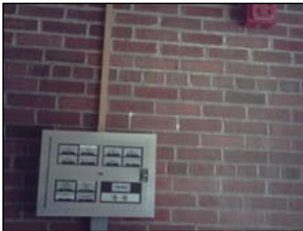
Fire Alarm Systems: Outdated System
