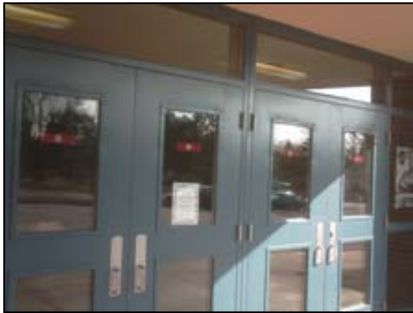
Communication and Security: Access Control
