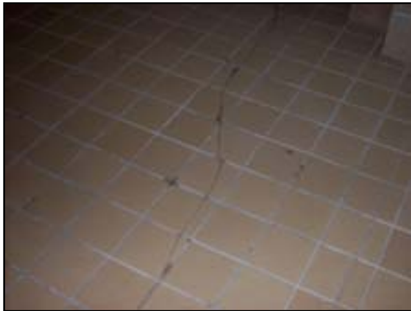
Floor Finishes: Replace Damaged Quarry Tile -
