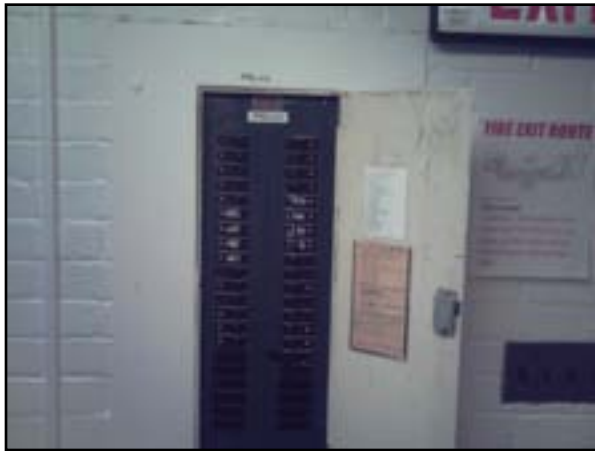
Electrical Distribution: Insufficient Capacity
