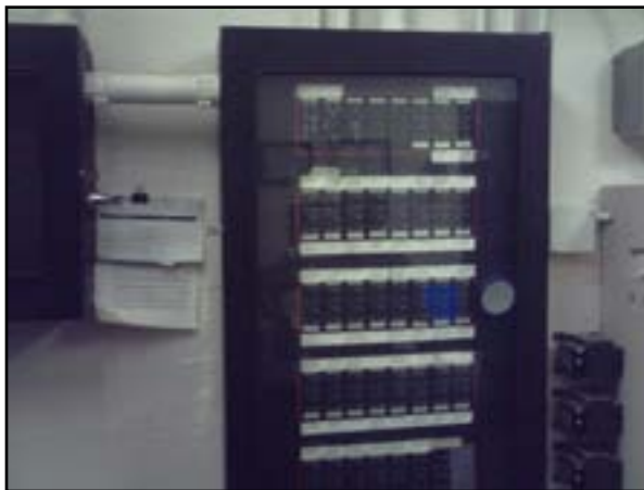
Fire Alarm Systems: Outdated System
