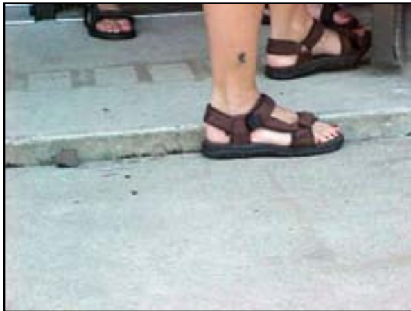
Site Improvements: Accessibility
