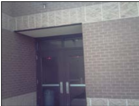
Communication and Security: Access Control
