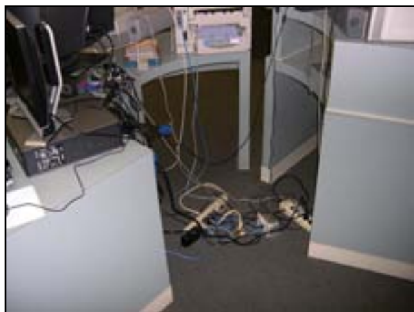
Wiring Devices: Insufficient Receptacles Wiring Devices: Insufficient Receptacles
