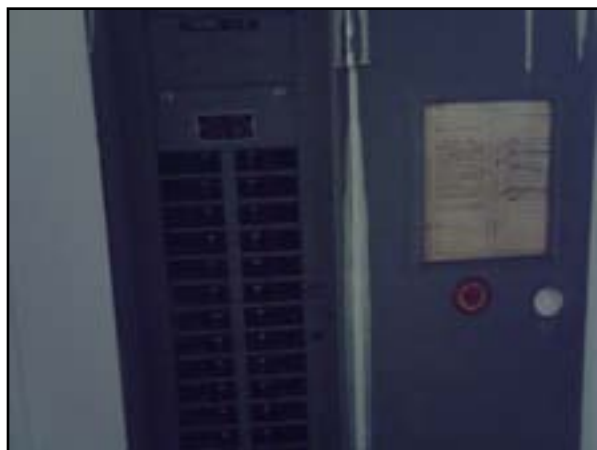
Electrical Distribution: Insufficient Capacity
