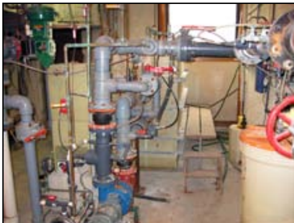
Aquatic Facilities: Filtration System Upgrade
