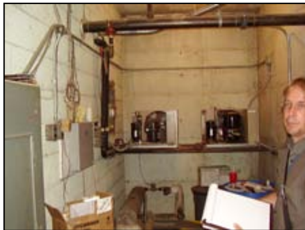
HVAC: Remote Condenser Heat Removal
