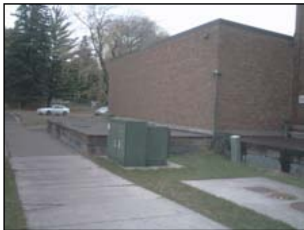
Emergency Power Distribution: Generator Backup
