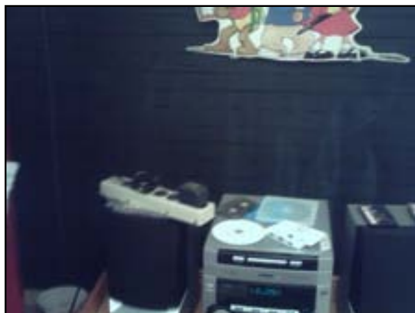
Wiring Devices: Insufficient Receptacles
