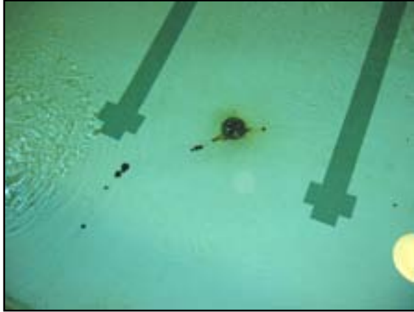
Aquatic Facilities: Deferred Maintenance Items
