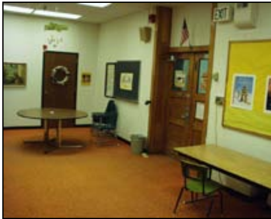
Floor Finishes: Replace All Carpet
