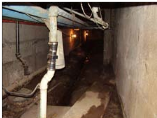
HVAC: Provide Negative Pressure in Crawlspace/Tunnels
