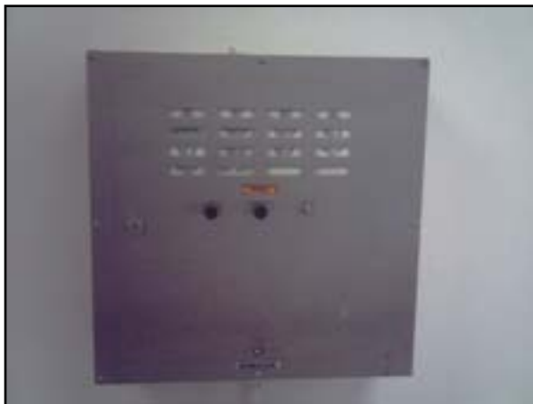
Fire Alarm Systems: Outdated System
