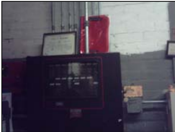
Fire Alarm Systems: Outdated System
