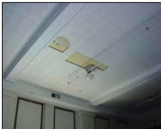
Ceiling Finishes: Repair Missing/Damaged Ceiling Tile
