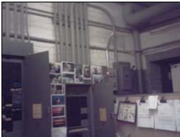
Electrical Service: Insufficient Capacity
