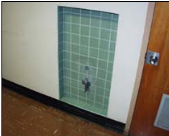
Wall Finishes: Repair Ceramic Tile at Drinking Fountain Recesses
