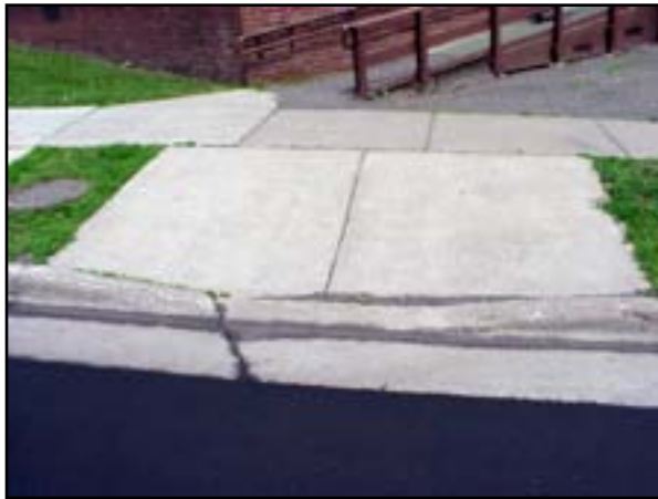
Site Improvements: Accessibility
