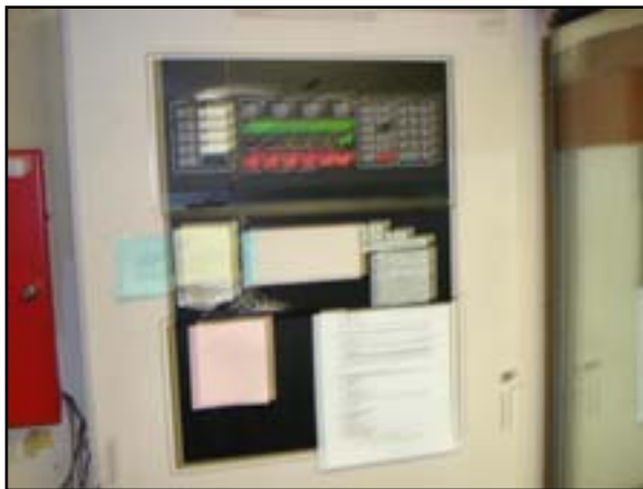
Fire Alarm Systems: Outdated System
