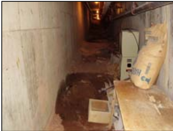
HVAC: Provide Negative Pressure in Crawlspace/Tunnels
