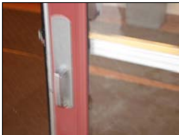
Communication and Security: Access Control
