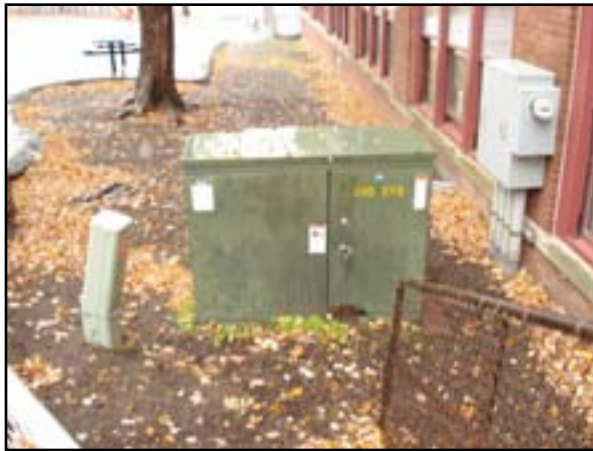
Emergency Power Distribution: Generator Backup
