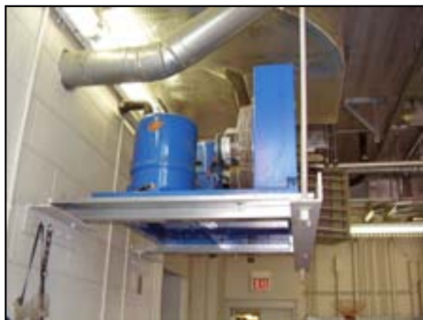
HVAC: Remote Condenser Heat Removal
