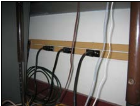
Wiring Devices: Insufficient Receptacles
