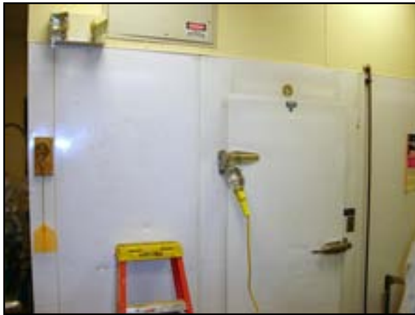
Other Equipment - Walk-In Cooler Condenser
