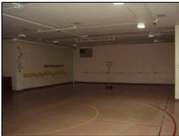
HVAC: Replace Ventilation to Gyms and Add Dehumidification to Cafeteria
