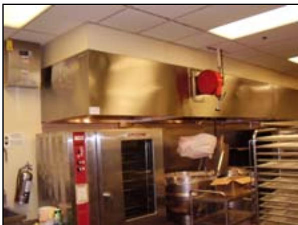
HVAC: Replace Kitchen Grease Exhaust Hood
