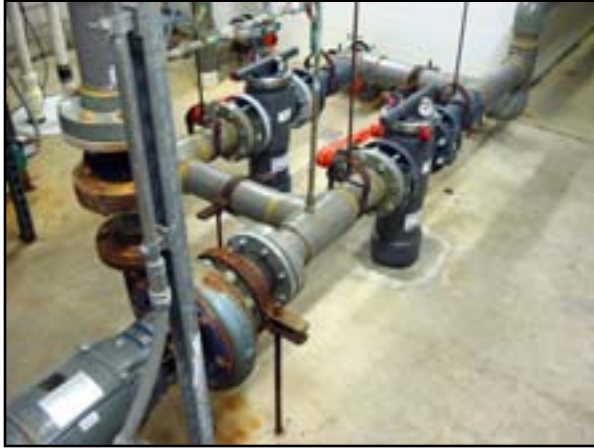
Aquatic Facilities: Deferred Maintenance Items
