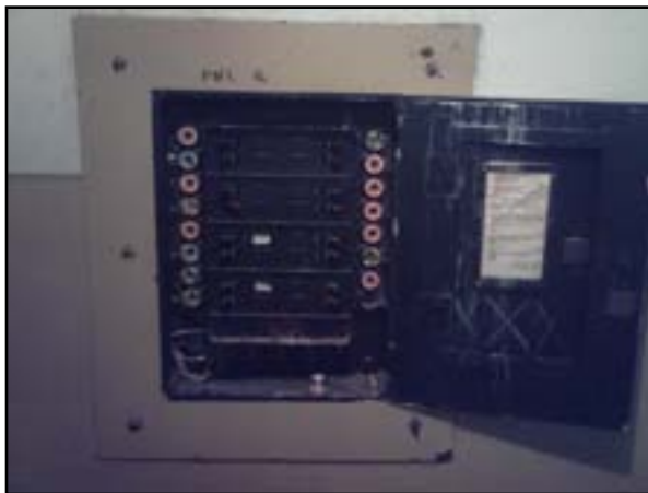
Electrical Distribution: Insufficient Capacity
