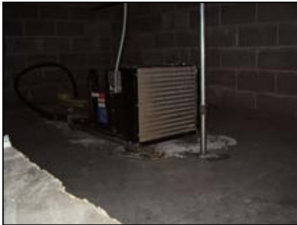
HVAC: Remote Condenser Heat Removal -
