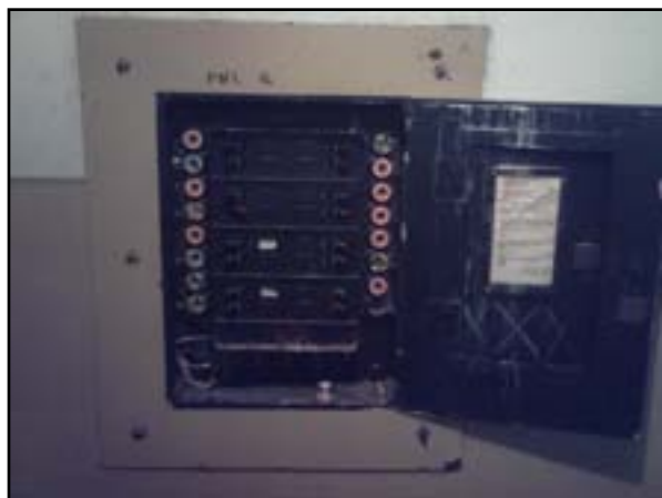
Electrical Distribution: Insufficient Capacity
