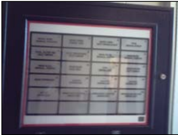
Fire Alarm Systems: Outdated System
