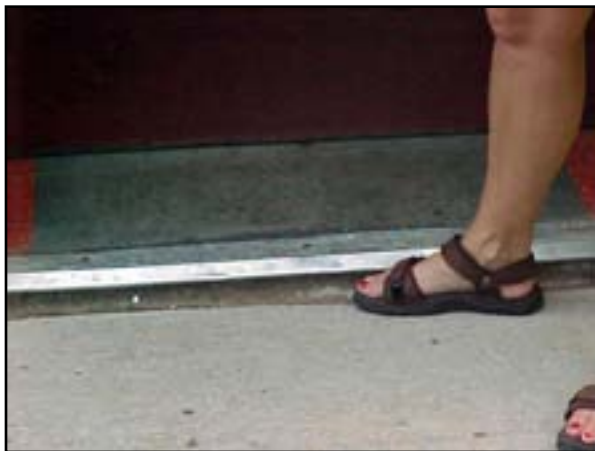
Site Improvements: Accessibility
