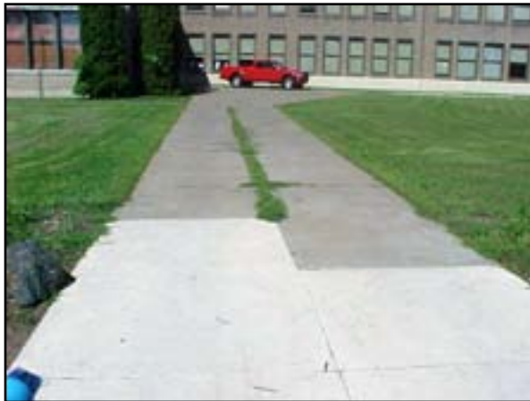
Site Improvements: Accessibility
