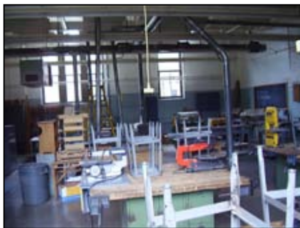
HVAC - Add Ventilation and Replace Wood Shop Dust Collector and Upgrade Weld Hood Exhaust
