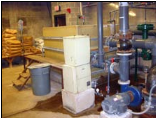
Aquatic Facilities: Filtration System
