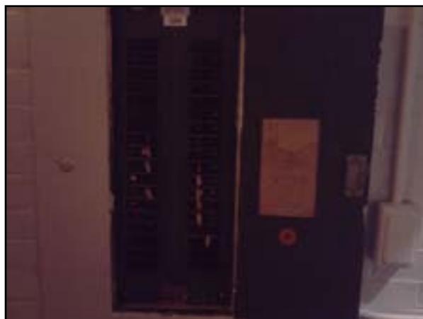
Electrical Distribution: Insufficient Capacity
