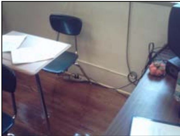
Wiring Devices: Insufficient Receptacles
