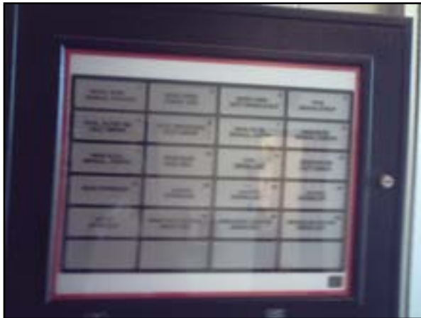
Fire Alarm Systems: Outdated System
