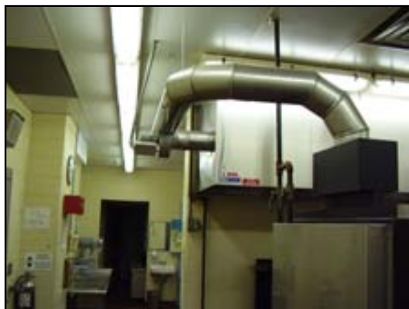
HVAC: Replace Kitchen Grease Exhaust Hood
