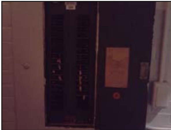
Electrical Distribution: Insufficient Capacity
