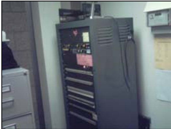
Communication and Security: Public Address and Sound System sound
