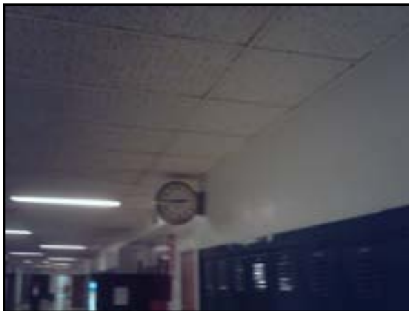
Communication and Security: Clock System
