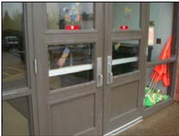
Communication and Security: Access Control
