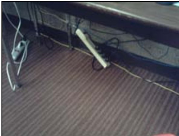
Wiring Devices: Insufficient Receptacles
