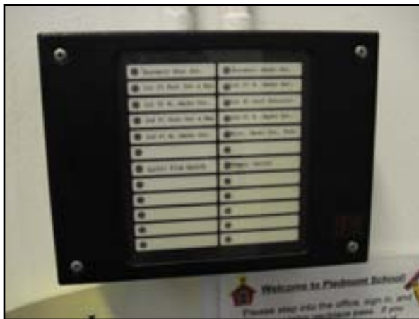
Fire Alarm Systems: Outdated System
