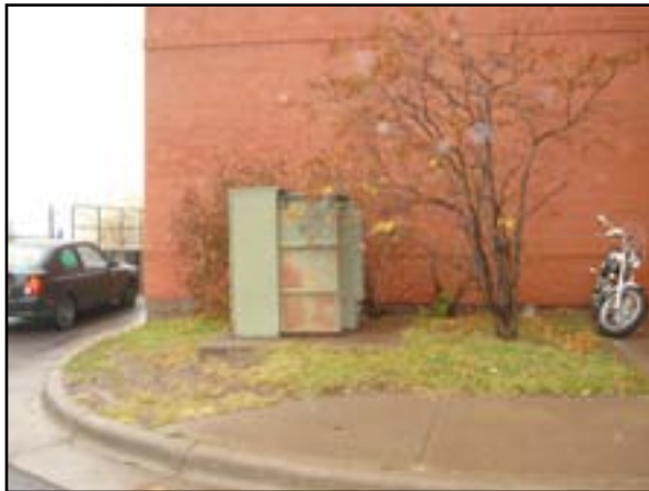
Emergency Power Distribution: Generator Backup
