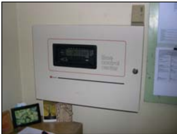
Communication and Security: Clock System
