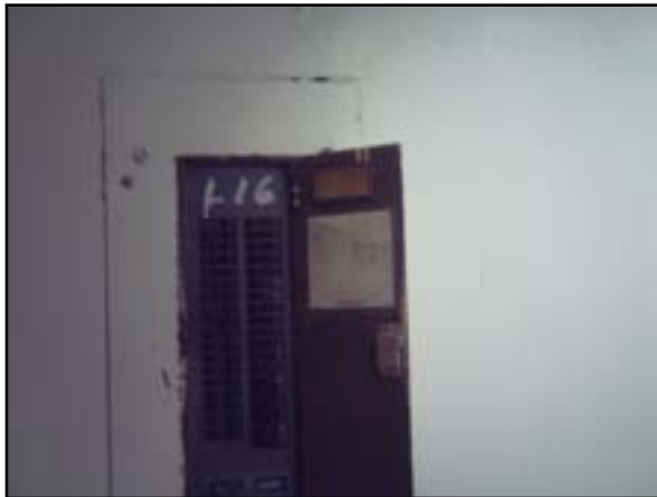
Electrical Distribution: Insufficient Capacity
