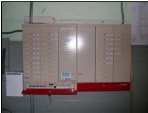
Fire Alarm Systems: Outdated System
