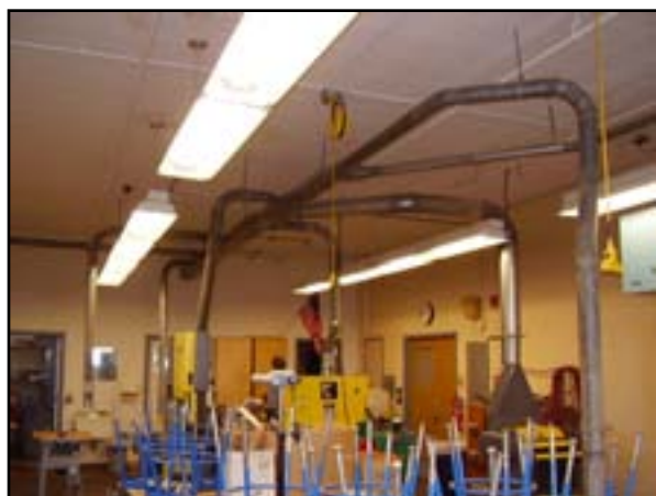
HVAC - Add Ventilation and Replace Wood Shop Dust Collector and Upgrade Weld Hood Exhaust
