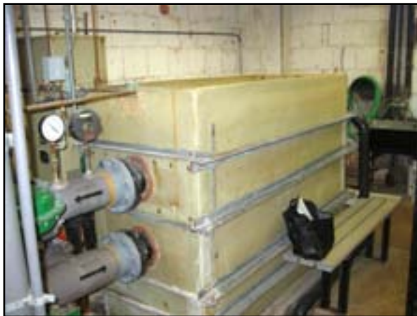
Aquatic Facilities: Filtration System
