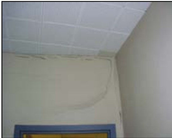
Superstructure: Wall Cracks
