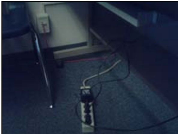
Wiring Devices: Insufficient Receptacles
