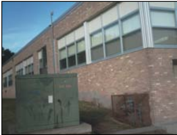
Emergency Power Distribution: Generator Backup
