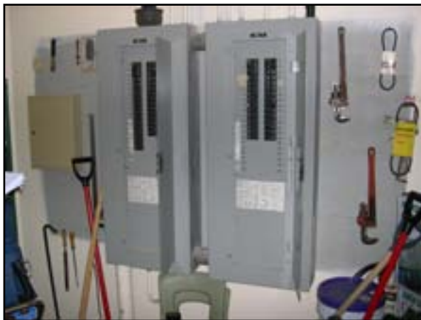
Electrical Distribution: Insufficient Capacity
