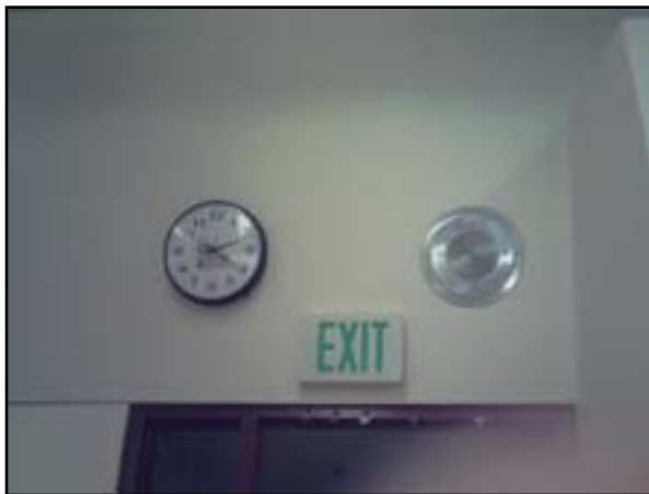
Communication and Security: Clock System
