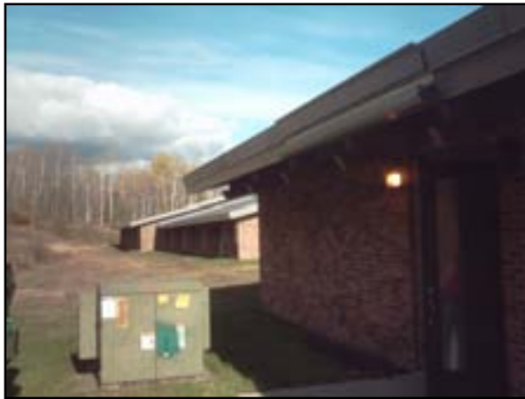
Emergency Power Distribution: Generator Backup
