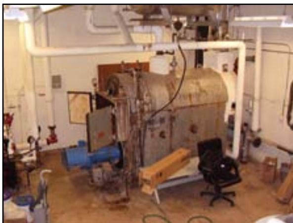
HVAC: Boiler Room Upgrades
