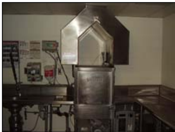
HVAC: Replace Dishwasher Exhaust Hood
