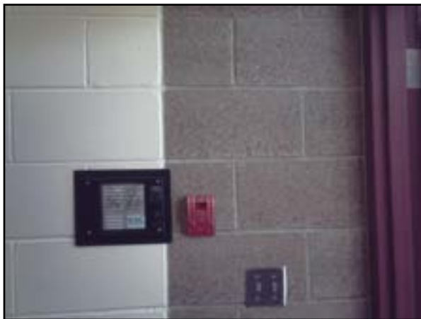
Fire Alarm Systems: Outdated System
