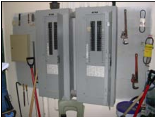
Electrical Distribution: Insufficient Capacity
