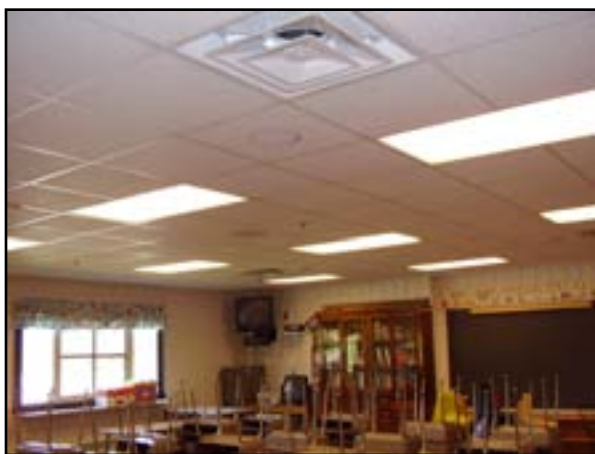
HVAC: Add Dehumidification to Classrooms
