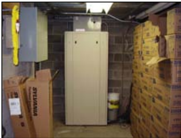
HVAC: Add Cooling Capability to IT Data Room
