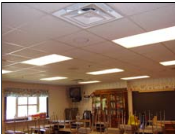
HVAC: Add Dehumidification to Classrooms
