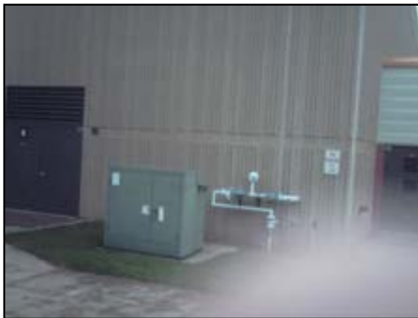
Emergency Power Distribution: Generator Backup
