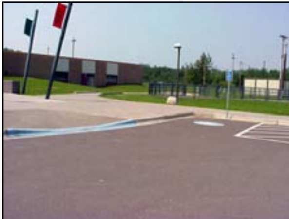
Site Improvements: Accessibility
