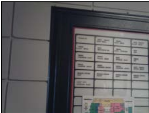
Fire Alarm Systems: Outdated System
