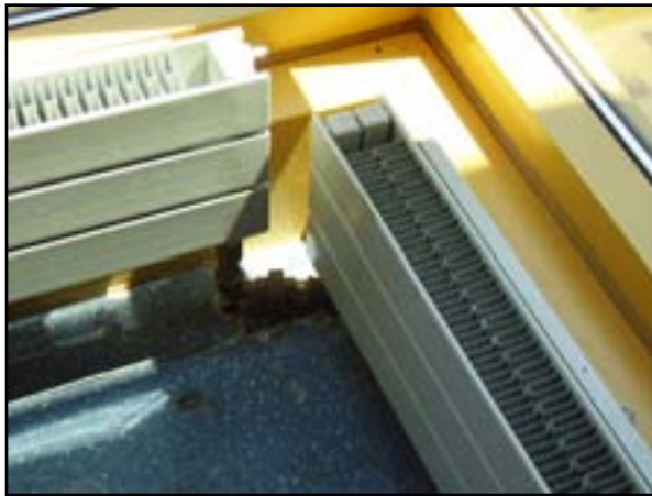
HVAC: Replace Leaking Underfloor Finned Tube Piping
