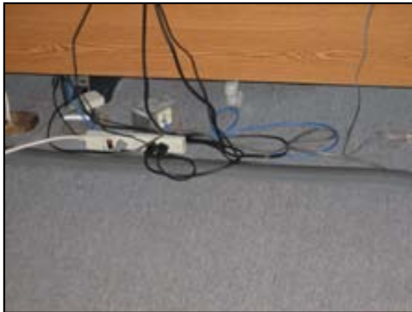
Wiring Devices: Insufficient Receptacles
