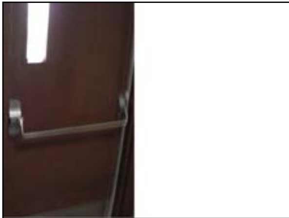
Communication and Security: Access Control
