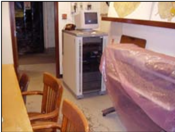
HVAC: Add Cooling Capability to IT Data Rooms
