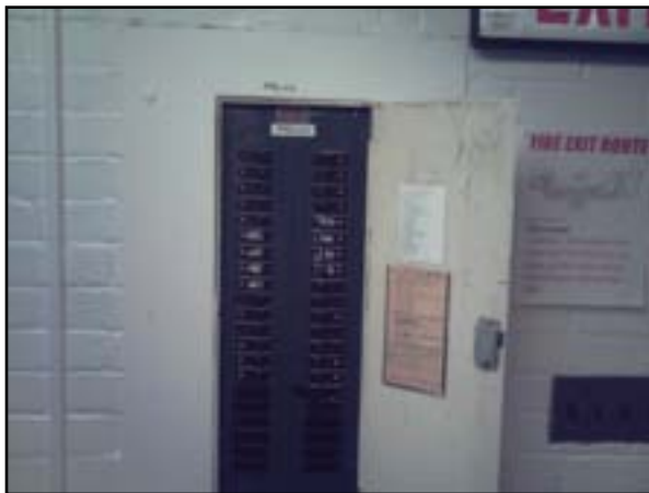
Electrical Distribution: Insufficient Capacity
