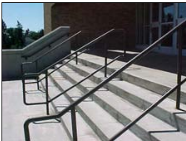
Site Improvements: Accessibility
