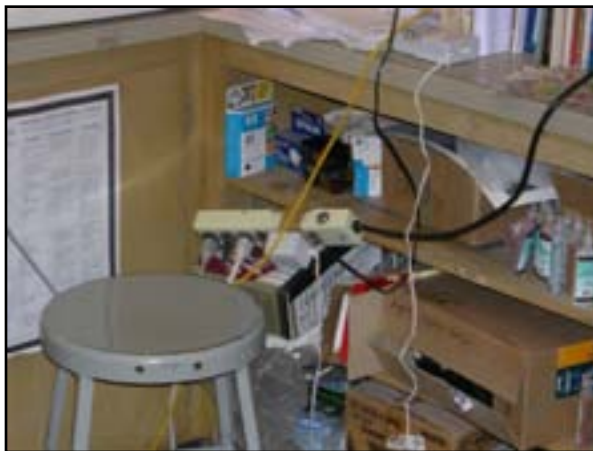
Wiring Devices: Insufficient Receptacles
