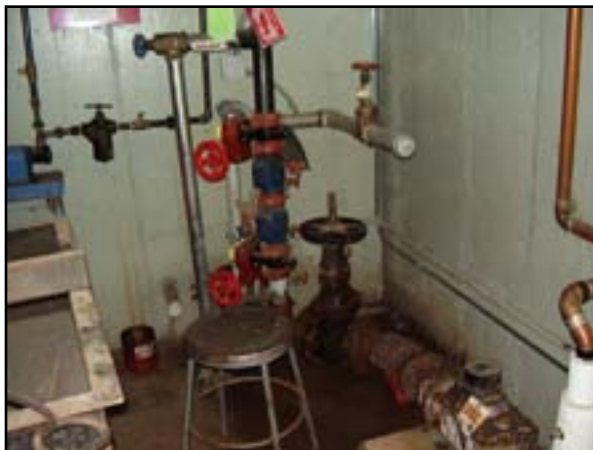
Fire Protection: Extend Fire Protection Sprinkler System
