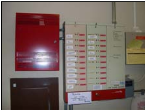
Fire Alarm Systems: Outdated System
