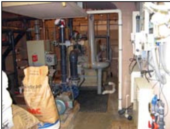
Aquatic Facilities: Filtration System Upgrade
